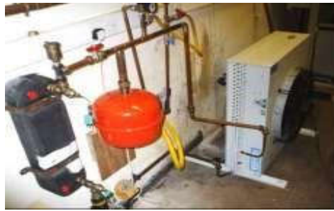
Figure 15. Shows the connections of the heat exchanger, water pump, heat rejection fan and expansion valve.
