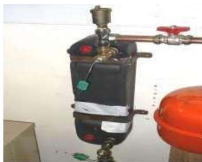
Figure 14. Shows the heat exchanger.
